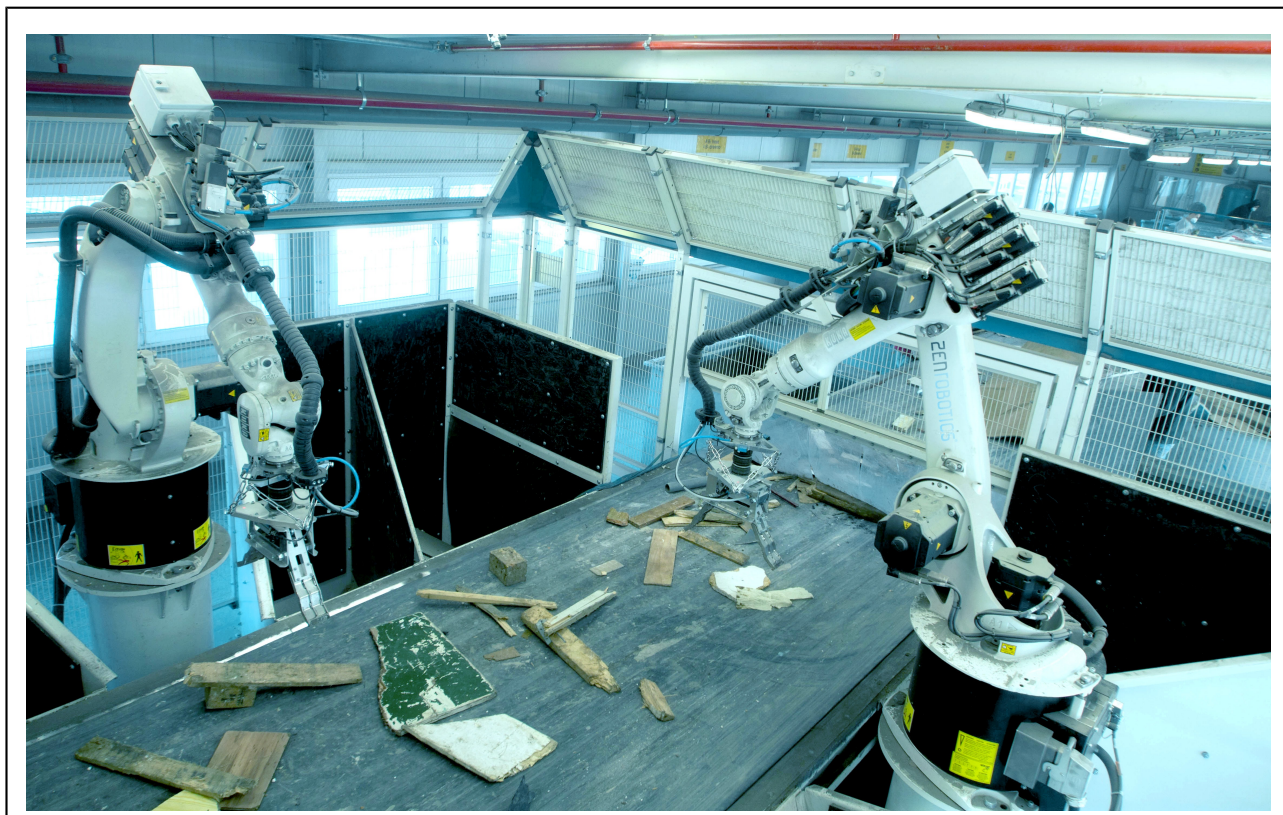
Figure 4: Retrofit ZRR Fast Picker system installation. (Image © ZenRobotics Ltd 2014. Used with permission.)
